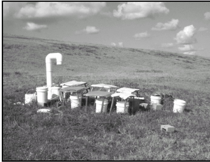
Fig. 3.12. Photo of Filters at LFG well.
