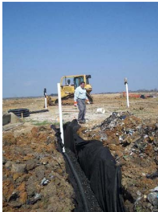
Fig. 3.7. (a) Placement of Tire Chips into geotextile wrap. (b) Perforated pipe laid into tire chips before being covered by more tire chips and wrapped in geotextile.
